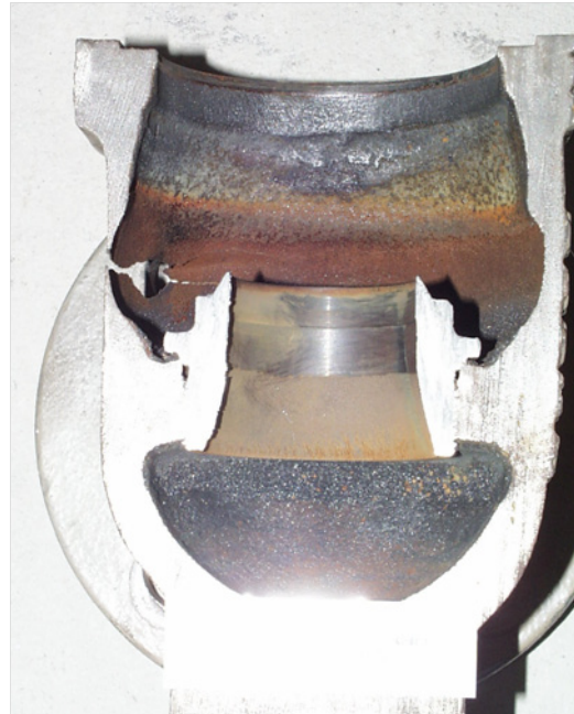
Figure 12.2.7.-1: Corrosion by a too high velocity of flow.
